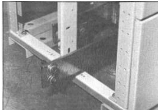
Fig. 14 Splice Plate Attached to Freedom 2100 Neutral Bus.
