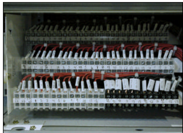
Fig. 16 Master Terminal Blocks
